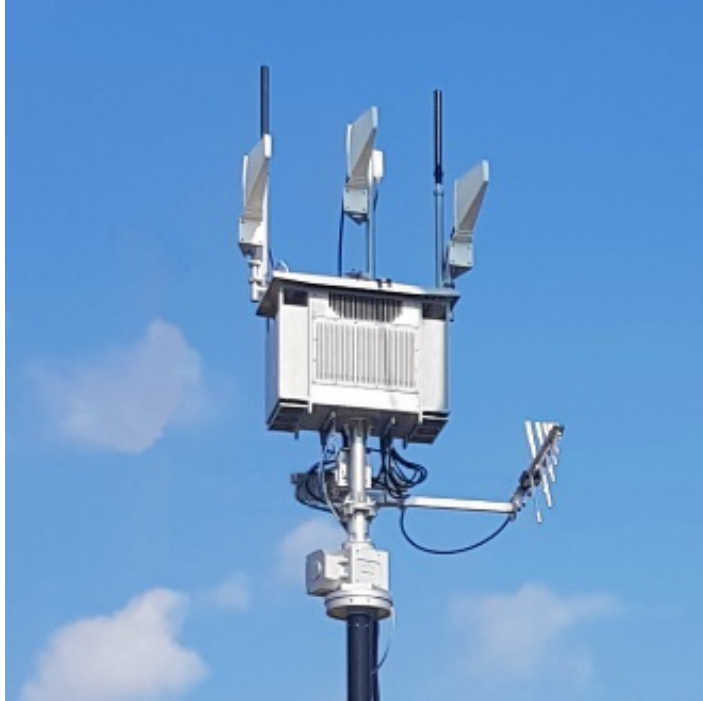
jamming transmitter antennas system
