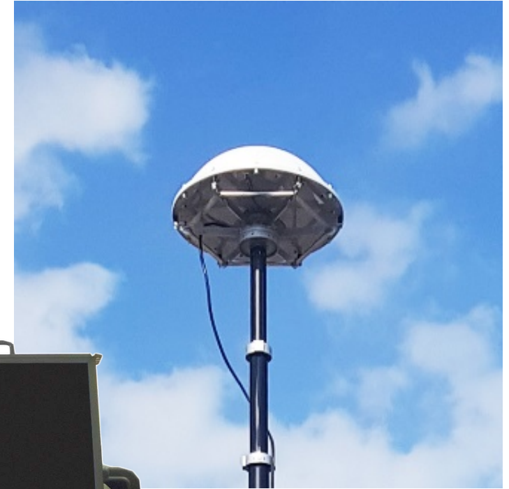
DF antenna system
